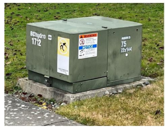
Pad Mount Transformer (PMT)
