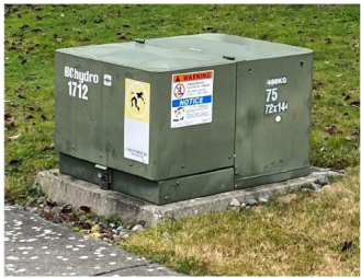
Pad Mount Transformer (PMT)
